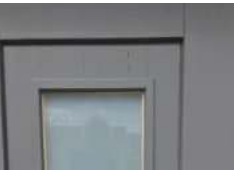
Crack formation, part 2
