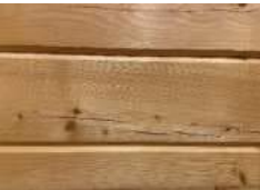
Crack formation, part 1
